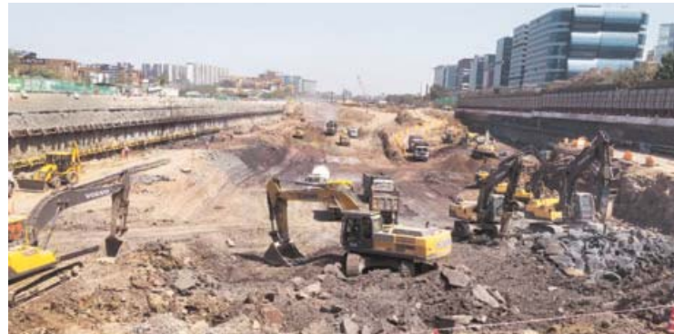
Excavation at Bandra Kurla Complex, where the underground Mumbai station of Mumbai-Ahmedabad high-speed rail is being built
